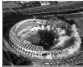
Like a lot of baseballs, the former home of the Atlanta Braves collapsed Saturday. (Courtesy 1994)
